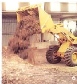
5. Biosolids processing —Design, contract management, and start-up of new biosolids processing facilities, including odor control, anaerobic digesters, dewatering equipment, and a 40-dry-tons-per-day pelletizing facility, will enable the Greater Lawrence Sanitary District (Mass.) to avoid costly sludge disposal.
