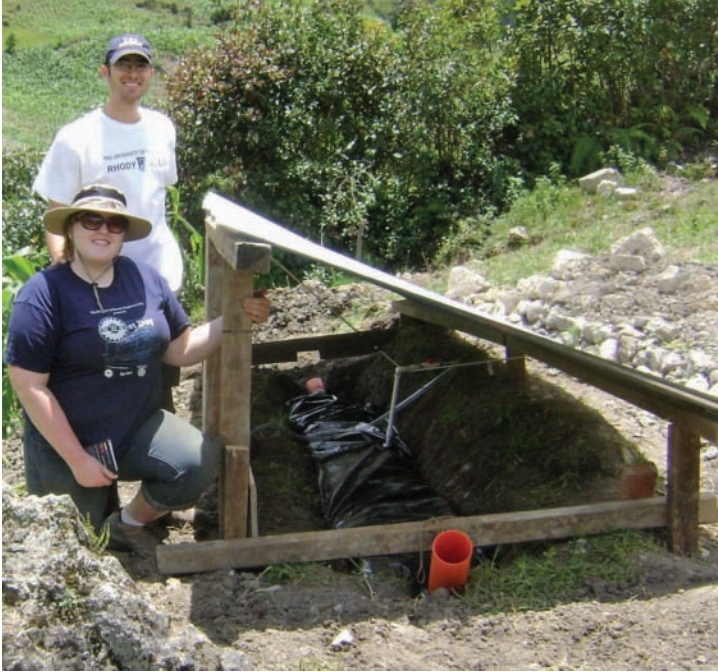
A 6-meter in diameter reactor is made from $100 worth of polyethylene and other materials purchased in San Mateo. A PVC fitting connects the biodigester to a gas bag.
